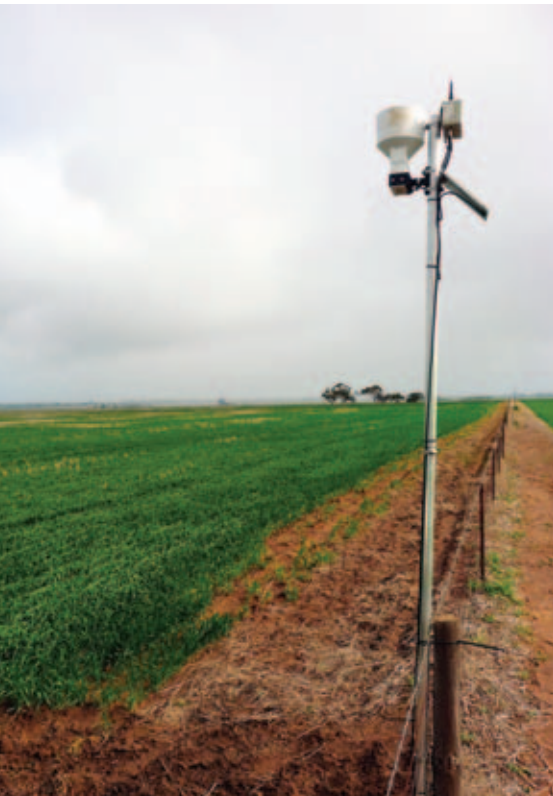
THIS MOISTURE PROBE INSTALLATION INCLUDES A RAIN GAUGE AND TELEMTRY THAT TRANSFERS THE MOISTURE DATA DIRECT TO A COMPUTER.
