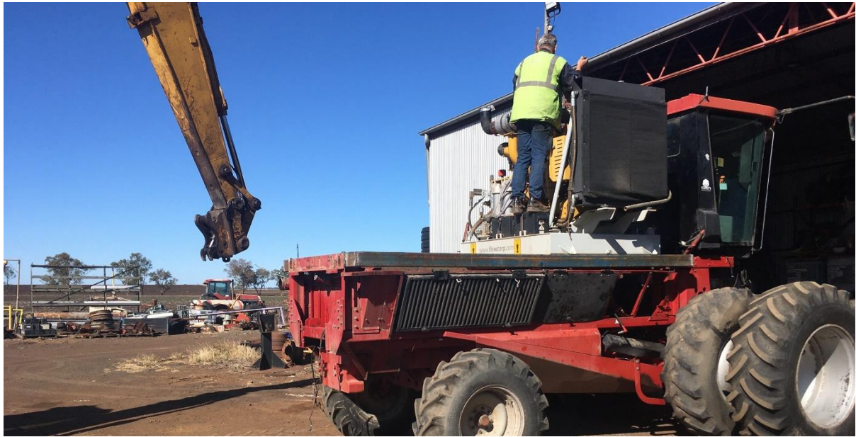
Figure 6: The 50,000 psi Flow Husky and diesel engine was fastened onto the redundant cotton picker chassis
